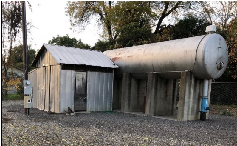
Figure 4 - Durham Irrigation District – Well #3
