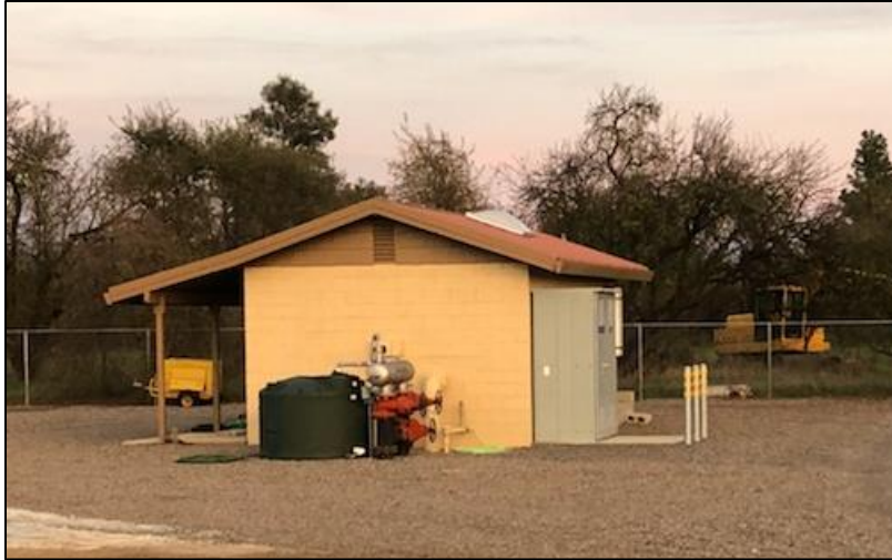
Figure 6 - Durham Irrigation District – Well #5
