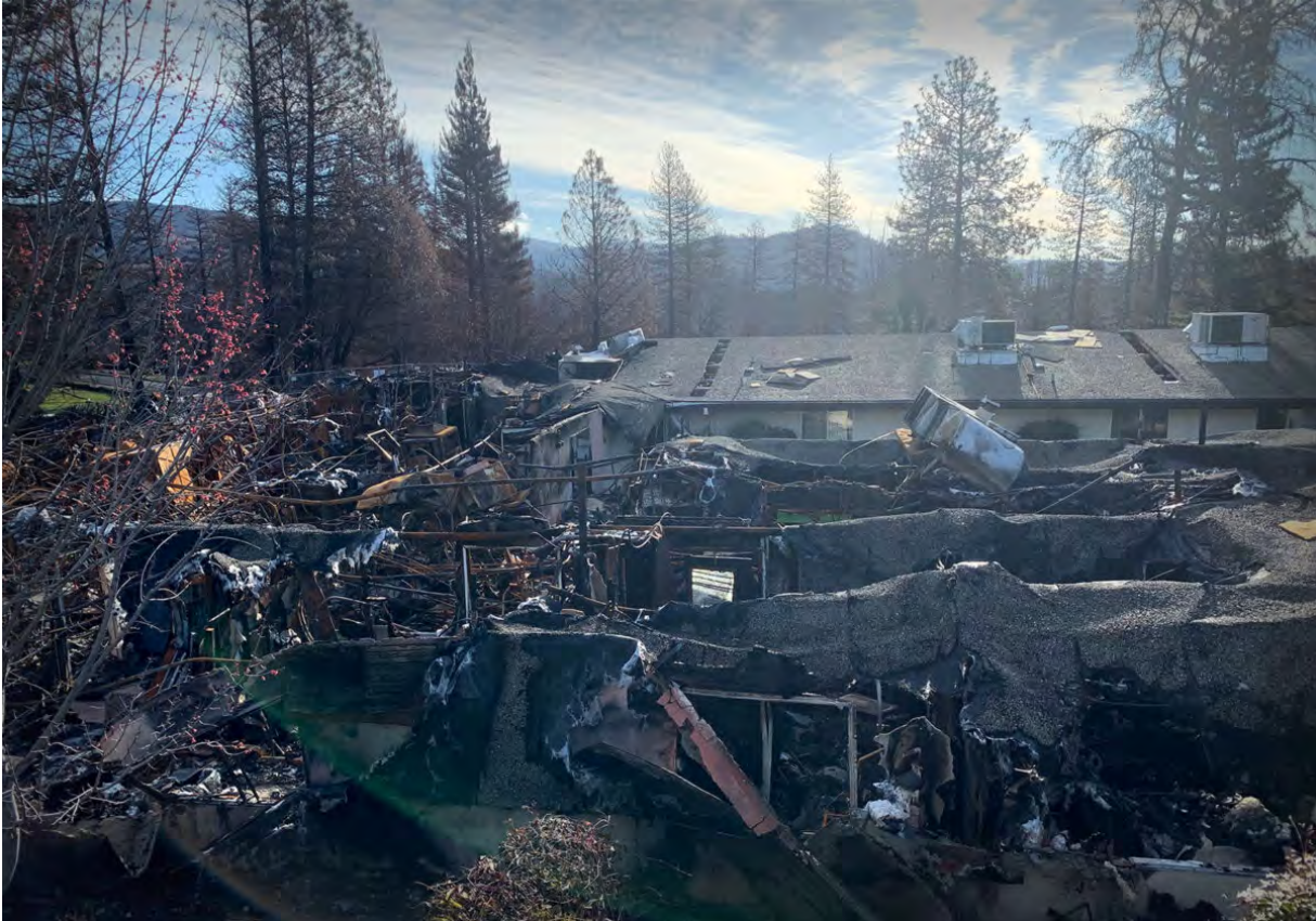
The collapsed roof of the Adventist Health Feather River Hospital's emergency room in March 2019, from a survey conducted by researchers studying the wildfire damage to structures < https://link.springer.com/article/10.1007/s11069-020-04197-0#Sec2 > . Erica Fischer, Oregon State University
